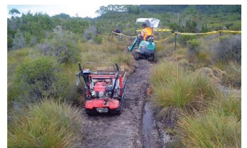
A mini-excavator and power wheelbarrow in action on the Frenchmans Cap Track works.
